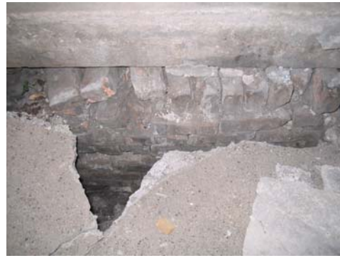
Defective Masonry Under Slab
