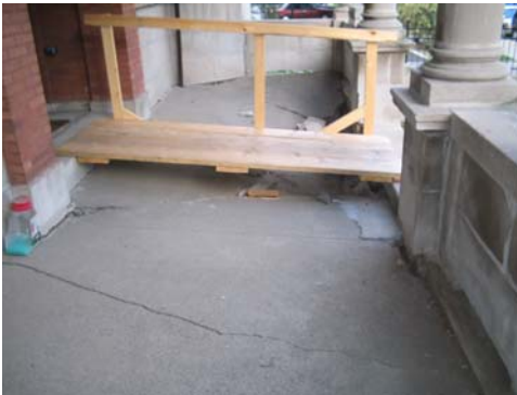
Defective Slab Cracking and Sinking
